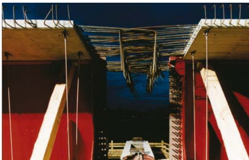
Fig. 11: Practical example: preparation for the concrete cross-beam over intermediate support – Oberhartmannsreuth Viaduct
