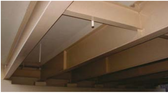
Fig. 19: Execution of detail of I-cross-beam welded to the web of the main girder
