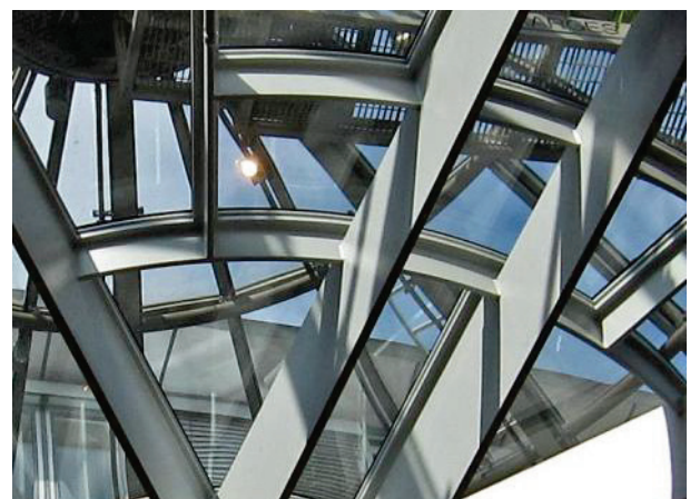
Fig. 3: Fire protection coatings, only a few millimetres thick and applied in line with the profile, emphasise the filigree nature of the structural steel design.
